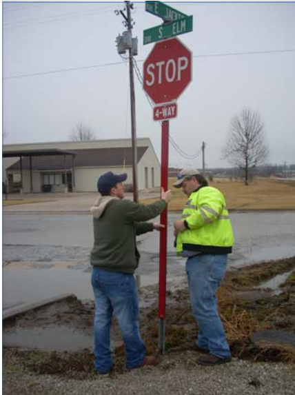
Marshfield City workers, Sam Rost and Greg Perryman install a sleeve post near the High School and Shook Elementary.
